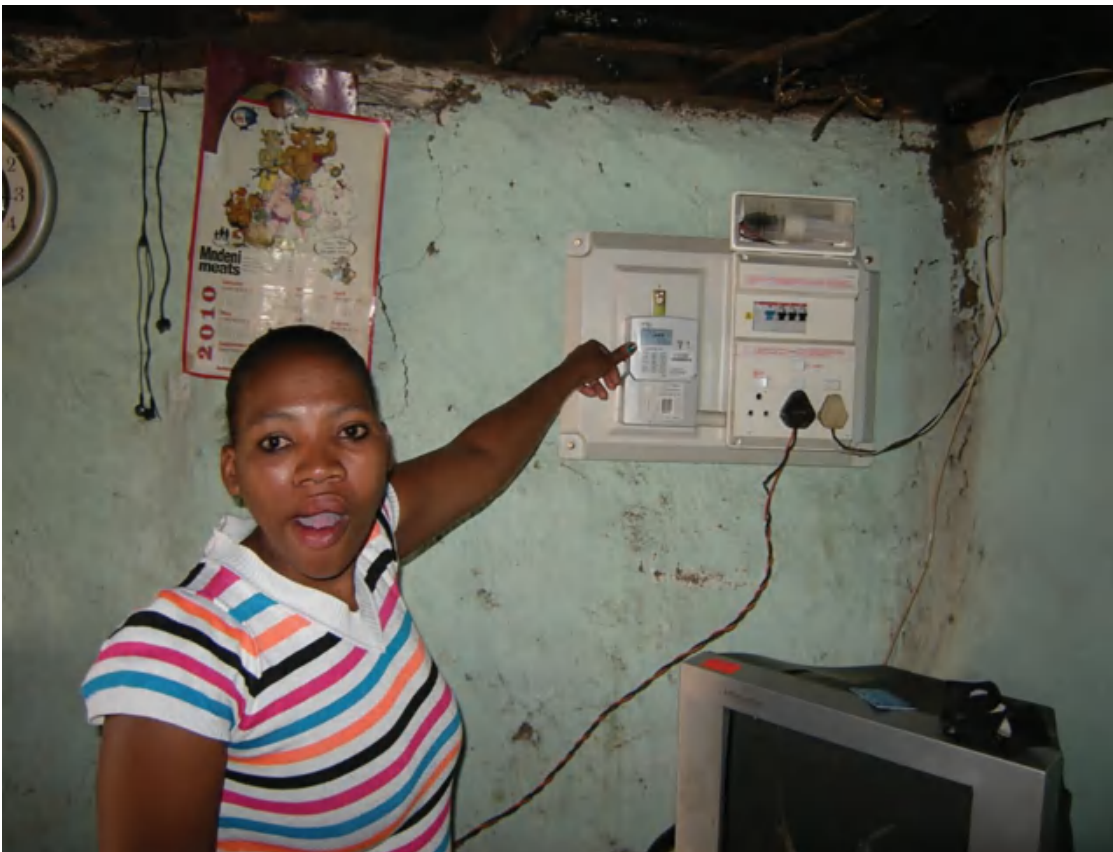
Individual electricity connection inside an informal settlement, South Africa
